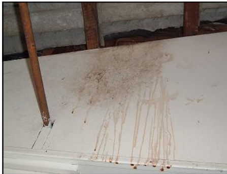
Possum urine stains on wall
